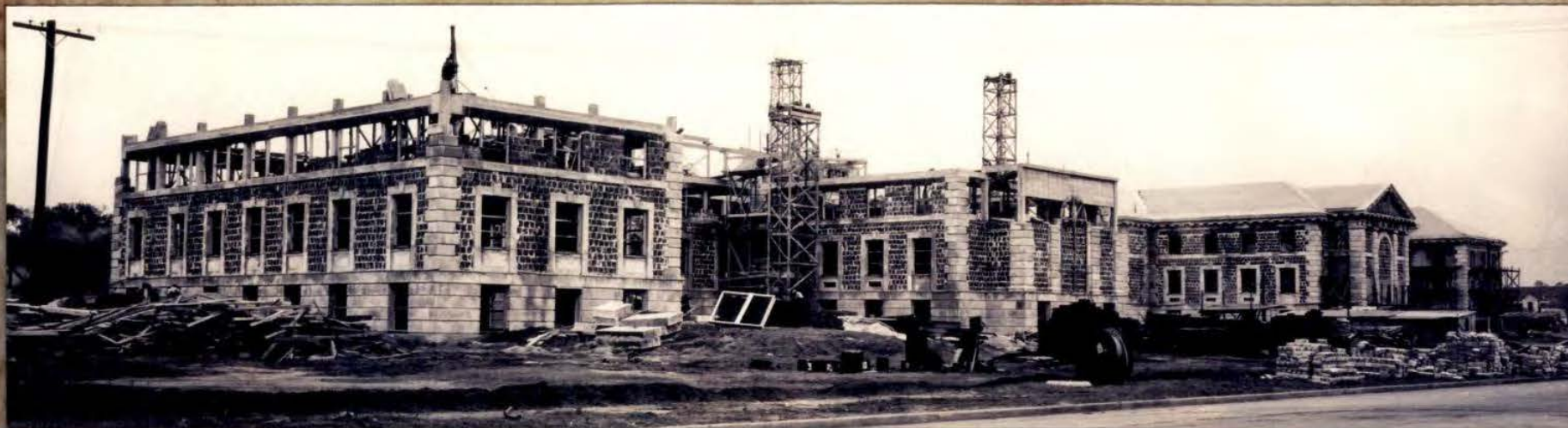
Rear view of The Infantry School under construction. Started April 6, 1934 and completed July 21, 1935, The Infantry School was built by the Dice-Schmidt Construction Company out of Chicago at a cost of $556,321.
